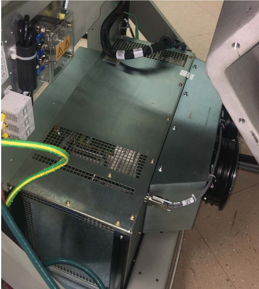
Figure 47 Stationary Power Inverter Fan and Air inlets/outlets
